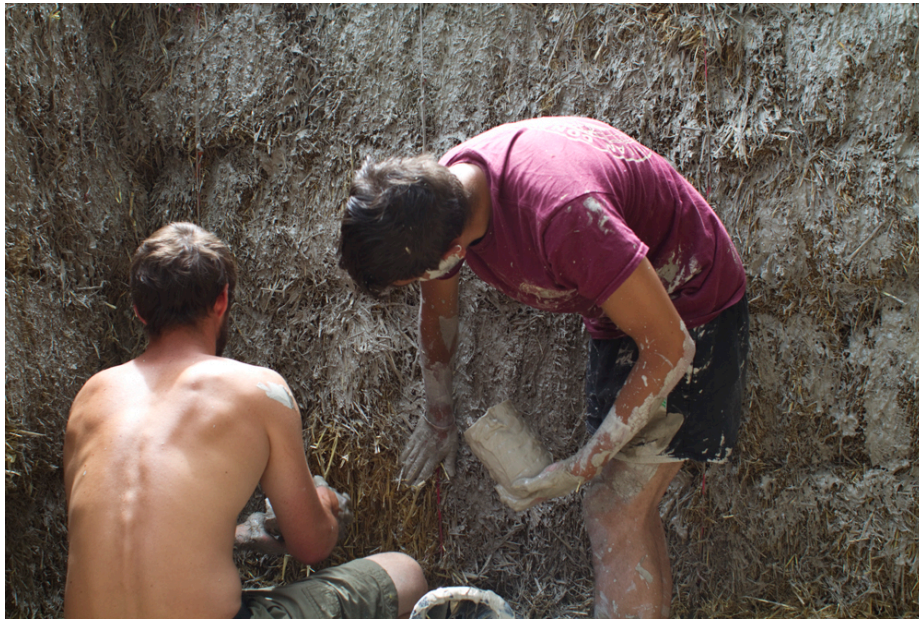
The straw needs a pure clay 'key' layer before applying the Cob
