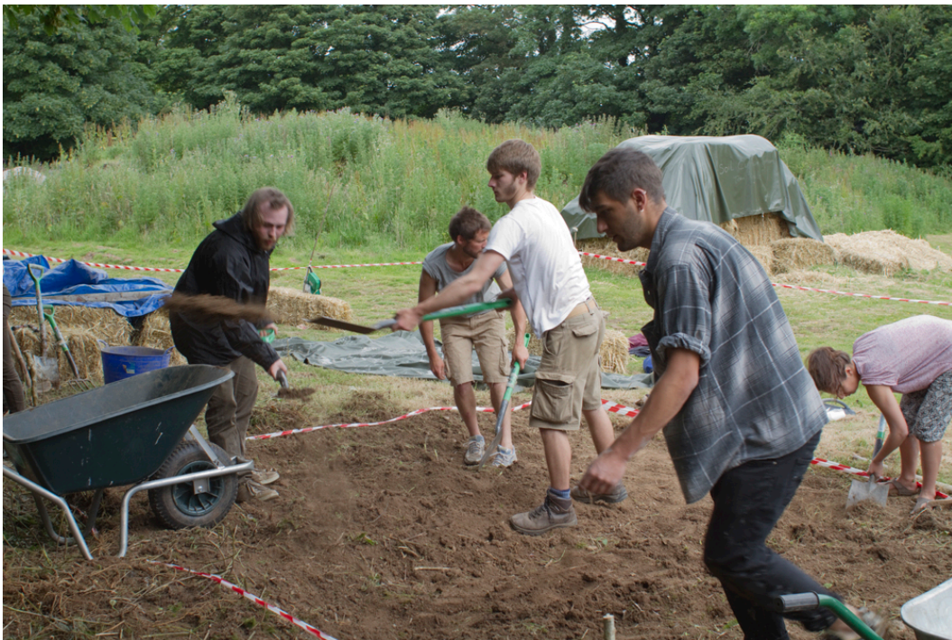
Clearing and leveling the site looking out for thistle and dandelion roots or anything else that may grow through the floor membrane. Marking out the footprint of the shed with the first layer of rammed earth tyres for the foundation plynth.
