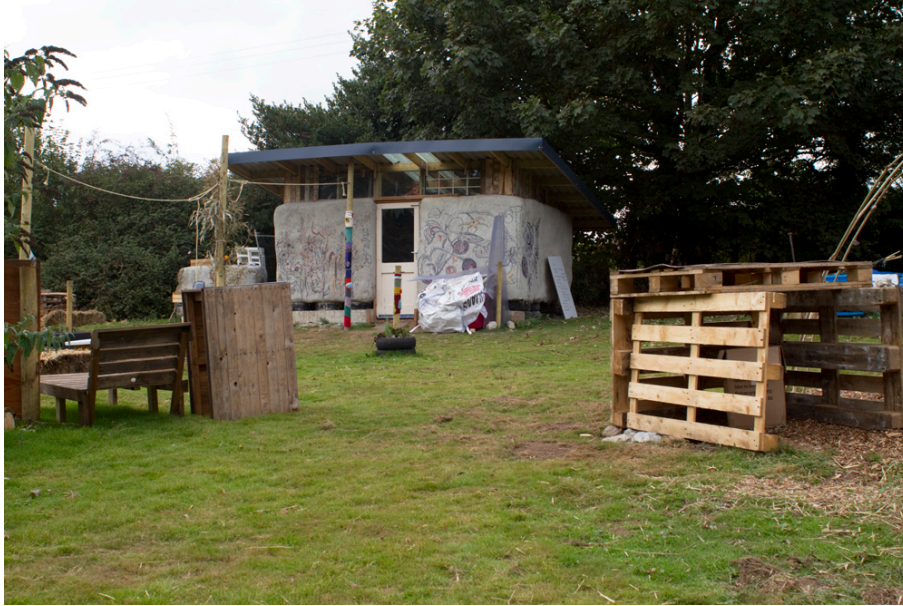
The completed shed waiting for a top coat of lime wash. Strawbale and Cob building project with RANE, Soil Culture Forum and the Green Living Project. Falmouth University, Penryn Campus, Cornwall
