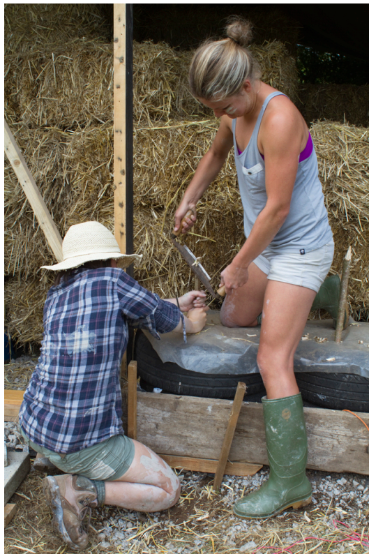
Preparing the base layer of hazel pins and connecting the bales to the plinth. Apart from a hedge trimmer used for trimming the strawbales the whole build was done with traditional hand tools.
