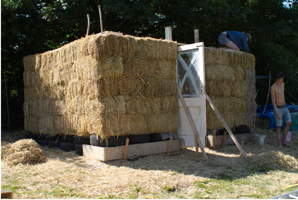
Using hazel pins and staples to hold the bales together, the straw walls go up in a morning.
