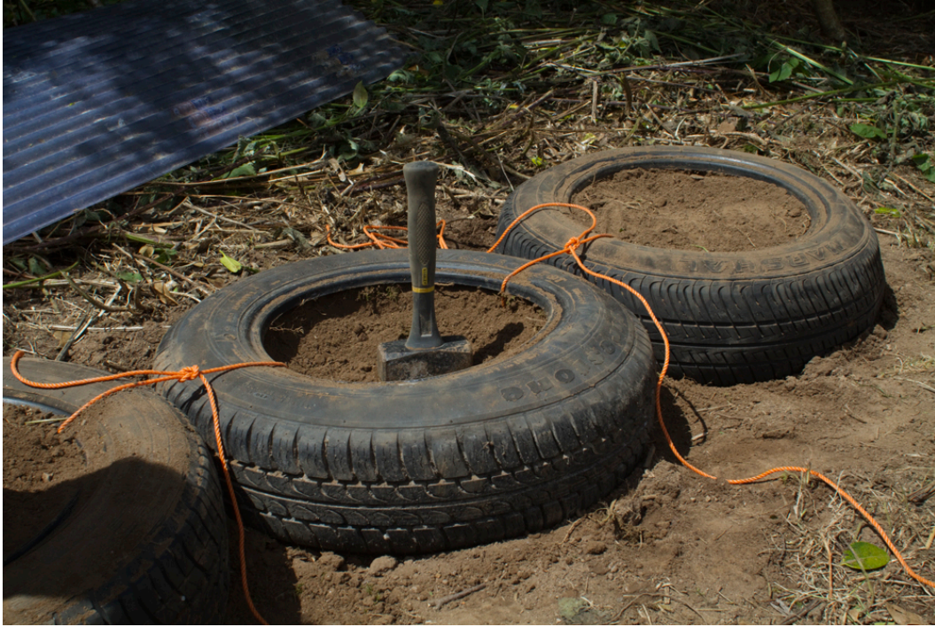
Marking out the footprint of the shed with the first layer of rammed earth tyres for the foundation plinth.
