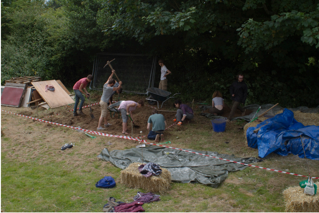
A large team of volunteers from the green living project make a start on the foundations
